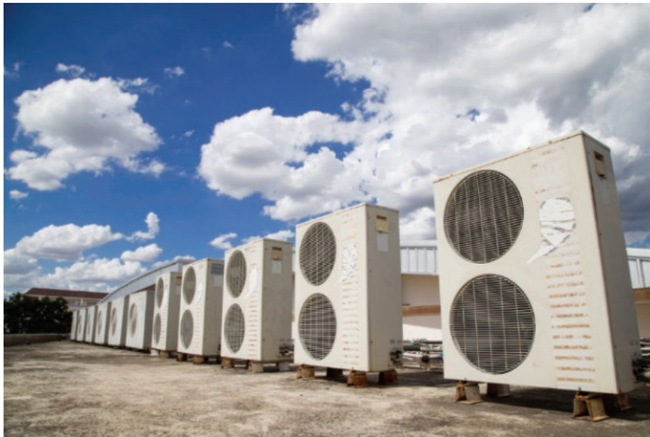
Figure 6 HVAC Rooftop Units. Image courtesy CanStockPhoto.com.
