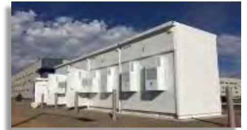
1 MW / 2 MWh battery system
