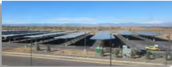
1.6 MW dc carport solar
